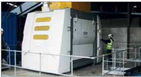
Application: Automotive shredder residue (ASR) Solution: TR3200 Location: Great Britain
